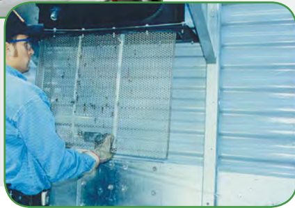
Inlet strainer inspection for Series 3000
